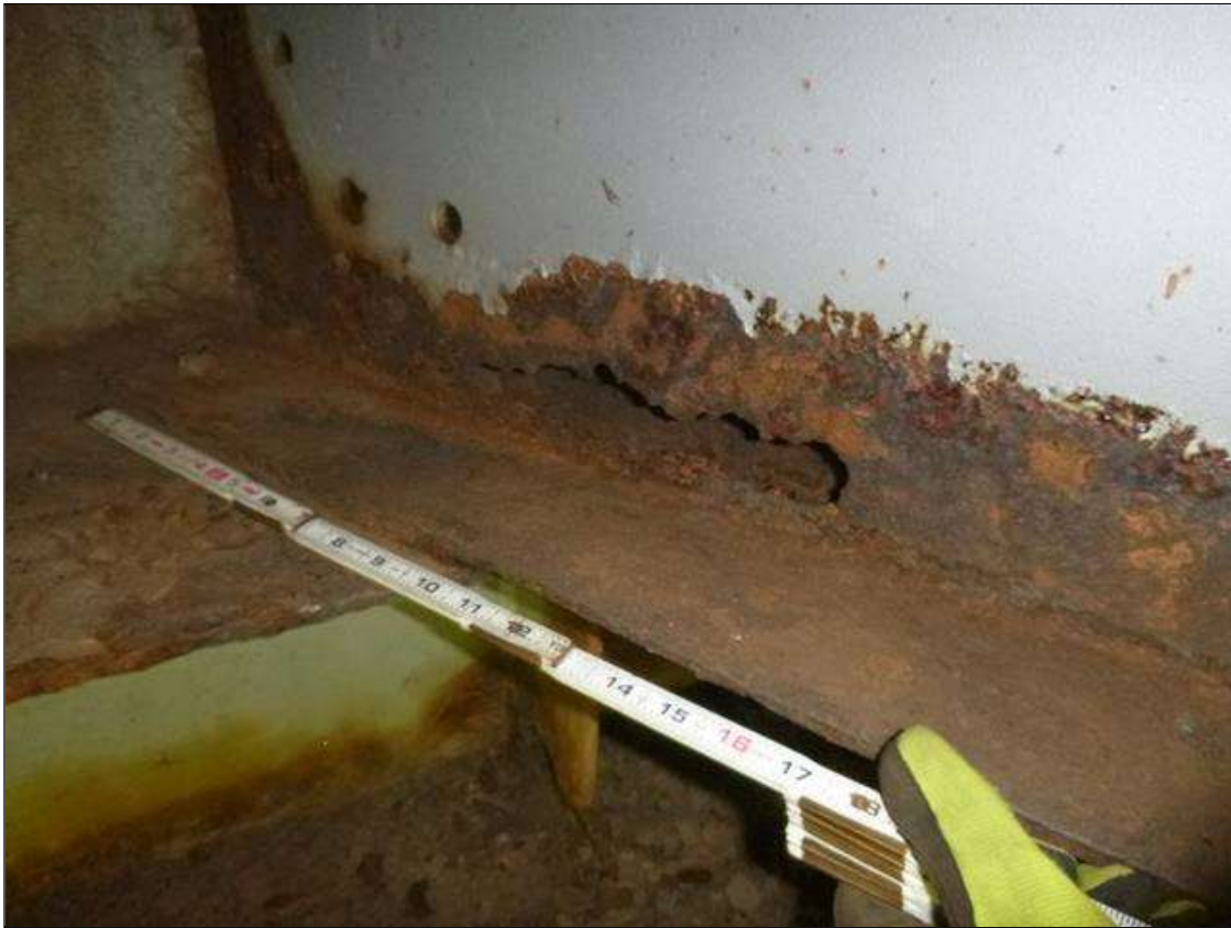
Span 1 Beam 6: [MUNICIPAL PROMPT ACTION REQUEST] AT END BENT 1, CORROSION WITH SECTION LOSS: BOTTOM FLANGE (0.35" AVERAGE REMAINING X 3'); LOWER WEB (3/16" AVERAGE REMAINING X 3' X UP TO 4") WITH RUST HOLE (12" X 1.5")
