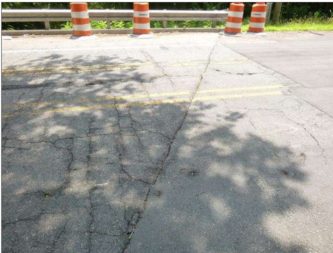
Span 1 Wearing Surface: at end bent 1, separation/ crack (1" x full width of roadway)
