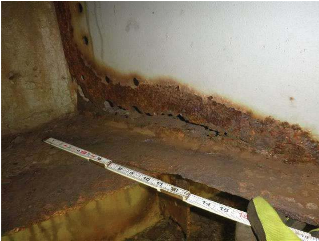
Span 1 Beam 8: [MUNICIPAL PROMPT ACTION REQUEST] AT END BENT 1, CORROSION WITH SECTION LOSS: BOTTOM FLANGE (0.40" AVERAGE REMAINING X 4'); LOWER WEB (3/16" AVERAGE REMAINING X 4' X UP TO 4") WITH RUST HOLE (16" X 3").
