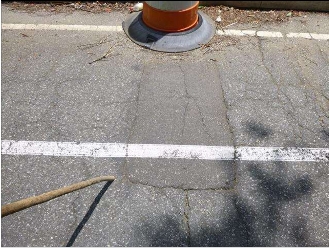
Span 2 Wearing Surface: at northbound lane near midspan, patched area (45" x 2') with cracks (up to 1/32")
