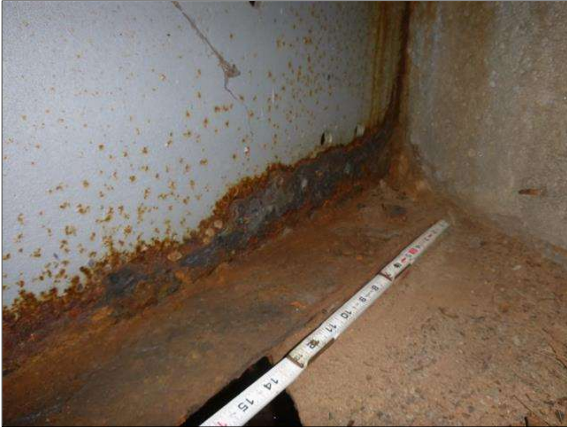
Span 3 Beam 4: [MUNICIPAL PROMPT ACTION REQUEST] AT END BENT 2, CORROSION WITH SECTION LOSS: BOTTOM FLANGE (0.45" AVERAGE REMAINING X 3.5'); LOWER WEB (1/4" AVERAGE REMAINING X 3.5' X UP TO 4").
