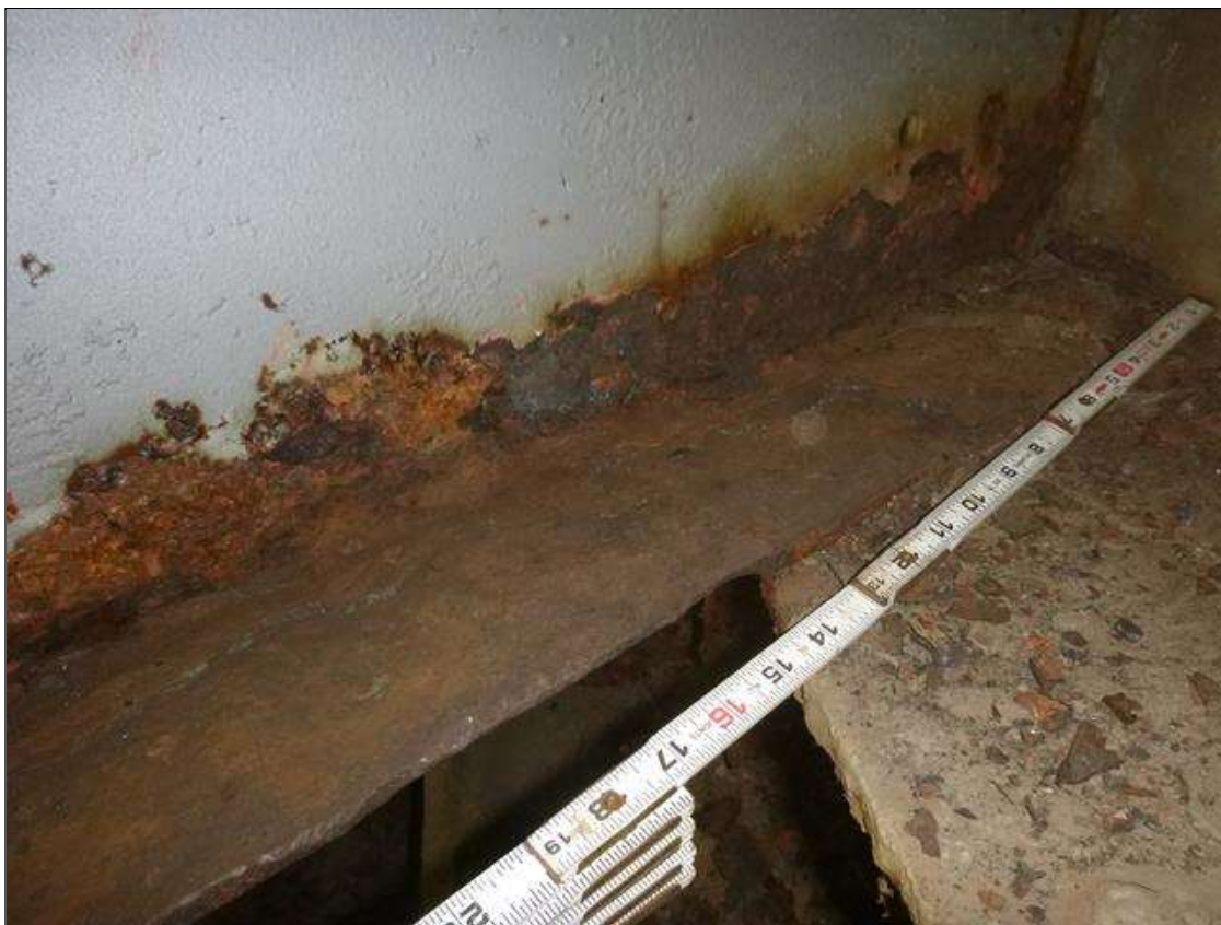
Span 1 Beam 5: [MUNICIPAL PROMPT ACTION REQUEST] AT END BENT 1, CORROSION WITH SECTION LOSS: BOTTOM FLANGE (AVERAGE 1/4" REMAINING FOR 1.5' LONG, THEN 0.40" AVERAGE REMAINING FOR NEXT 1.5' LONG'); LOWER WEB (3/16" AVERAGE REMAINING X 2.5' X UP TO 3.5")
