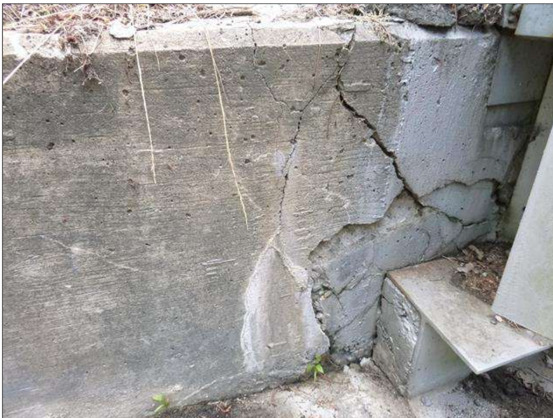
End Bent 2 Abutment: northwest wingwall adjacent to beam 1, spall/ delamination (3' x 2.5' x up to 2" deep) with cracks (up to 1/4") with efflorescence buildup
