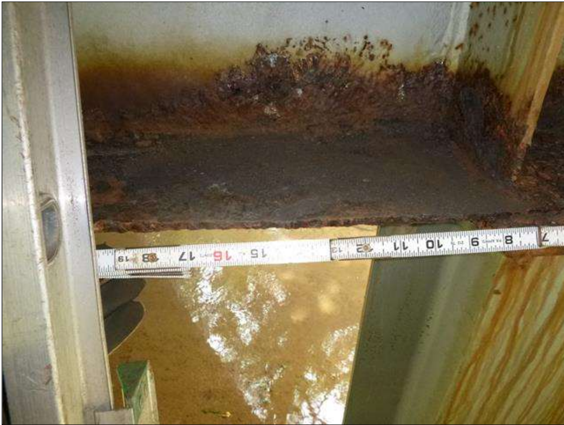
Bent 2 Cap 1: [MUNICIPAL PROMPT ACTION REQUEST] north face below beam 3, corrosion with section loss: bottom flange (0.35" average remaining x 5.5" x 5'); lower web (0.43" average remaining x 3' x 2.5")
