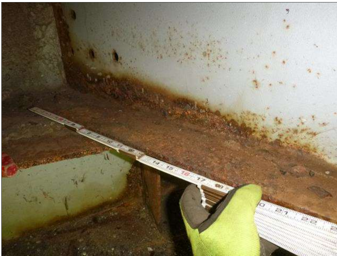
Span 1 Beam 9: [MUNICIPAL PROMPT ACTION REQUEST] AT END BENT 1, CORROSION WITH SECTION LOSS: BOTTOM FLANGE (0.45" AVERAGE REMAINING X 2'); LOWER WEB (1/4" AVERAGE REMAINING X 20" X 2.5")
