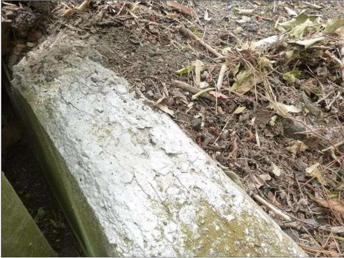
End Bent 1 Abutment: southwest wingwall adjacent to deck, spall (9" x 7" x 2.5" deep)
