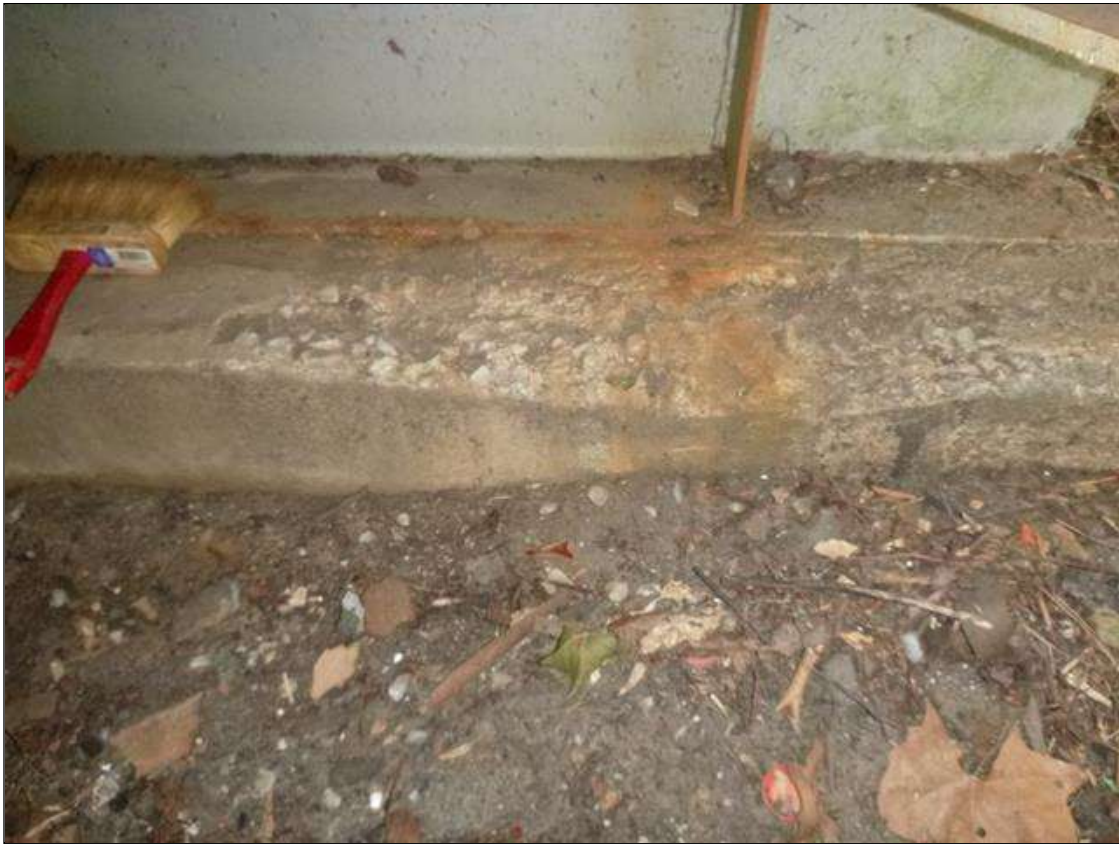
End Bent 1 Concrete Cap 1: 31" X 7" X 1 1/2" DEEP SPALL IN TOP OF CAP BENEATH BEAM 1
