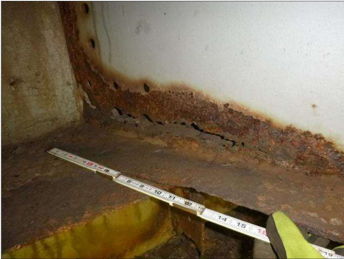
Span 1 Beam 8: [MUNICIPAL PROMPT ACTION REQUEST] AT END BENT 1, CORROSION WITH SECTION LOSS: BOTTOM FLANGE (0.40" AVERAGE REMAINING X 4'); LOWER WEB (3/16" AVERAGE REMAINING X 4' X UP TO 4") WITH RUST HOLE (16" X 3").
