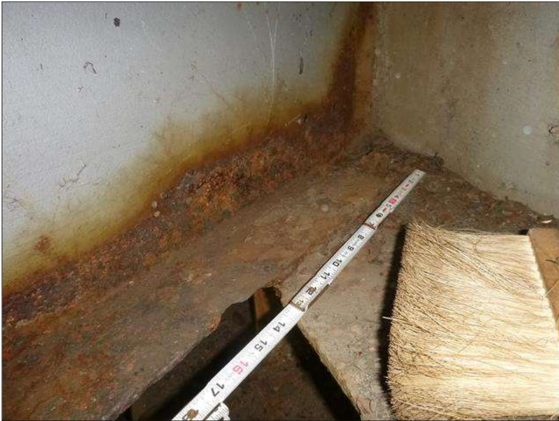
Span 1 Beam 3: [MUNICIPAL PROMPT ACTION REQUEST] AT END BENT 1, CORROSION WITH SECTION LOSS: BOTTOM FLANGE (1/4" REMAINING FOR 1.5' LONG, THEN 0.45" AVERAGE REMAINING FOR NEXT 2' LONG); LOWER WEB (1/4" AVERAGE REMAINING X 4' X 3")
