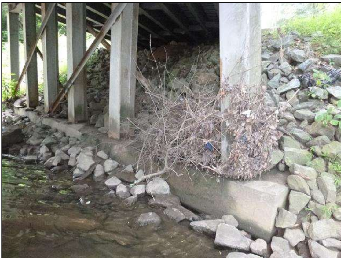
AT BENT 1, APPROXIMATELY 1 CUBIC YARD OF DRIFT HAS COLLECTED AGAINST THE PILES
