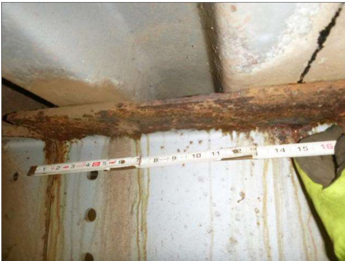
Span 1 Beam 4: [MUNICIPAL PROMPT ACTION REQUEST] at bent 1, top flange, corrosion with section loss (0.38" average remaining x 2')
