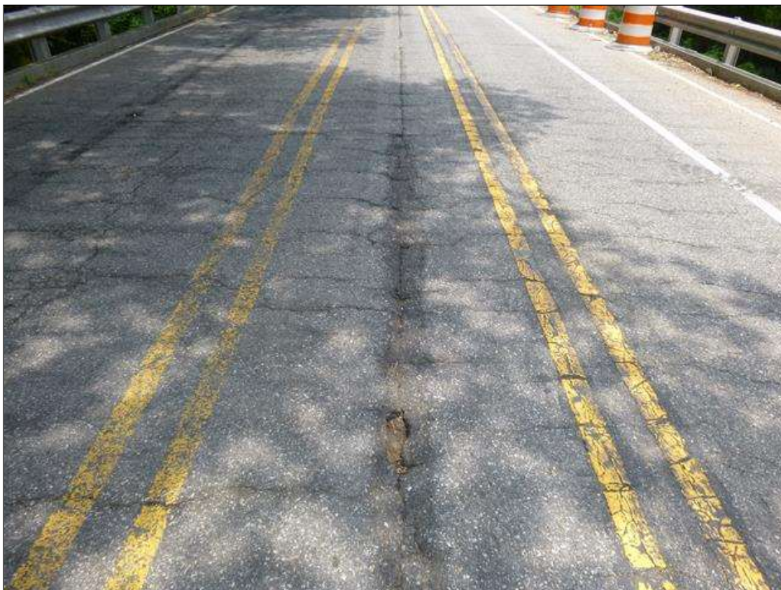
Span 1 Wearing Surface: at southbound lane, 2' from end bent 1, area of breaking up asphalt (14.5' x 6" x 1" deep)
