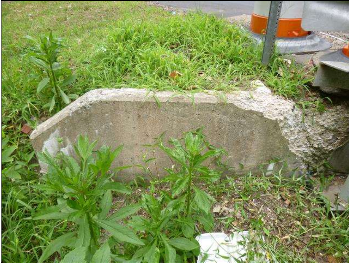
End Bent 1 Abutment: [MUNICIPAL PROMPT ACTION REQUEST] SOUTHEAST WINGWALL ADJACENT TO CURB, SPALL (2.5' X 1.5' X 3" DEEP) WITH EXPOSED RUSTED REBAR. THE CONCRETE SHOWS SIGNS OF ALKALAI SILICA REACTION.
