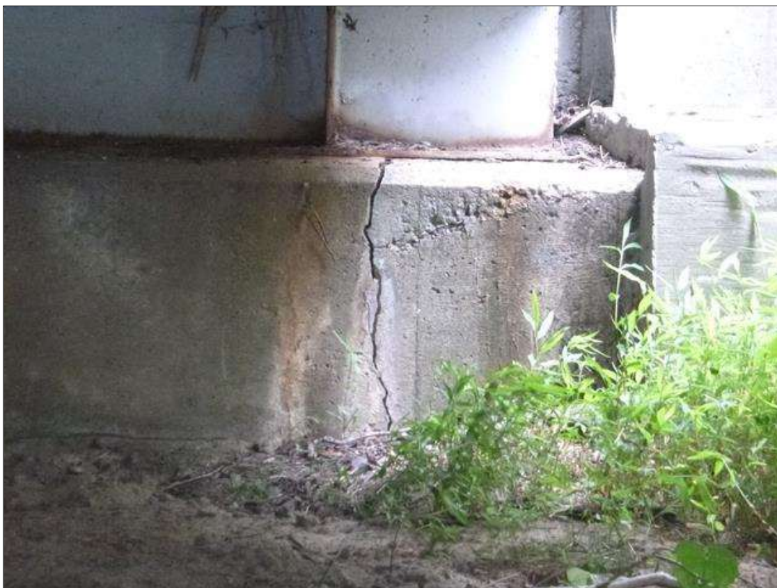
End Bent 2 Concrete Cap 1: concrete cap below beam 10, vertical cracks (up to 3/16" x full height) with efflorescence buildup
