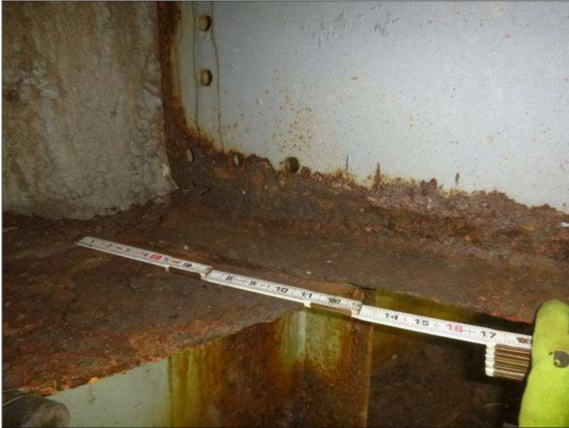
Span 3 Beam 8: [MUNICIPAL PROMPT ACTION REQUEST] AT END BENT 2, CORROSION WITH SECTION LOSS: BOTTOM FLANGE (0.375" AVERAGE REMAINING X UP TO 4'); LOWER WEB (1/8" AVERAGE REMAINING X 3" X UP TO 6" LONG WITH PERFORATIONS, THEN 3/16" REMAINING IN LOWER 3" OF THE WEB FOR THE NEXT 3.5' LONG)
