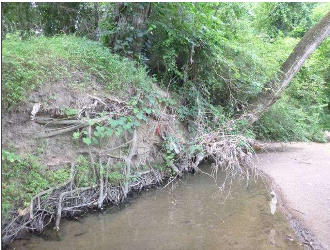
UPSTREAM AND DOWNSTREAM OF THE STRUCTURE THERE IS LOSS OF VEGETATION WITH EXPOSED ROOTS AND SLOUGHING UP TO 10' HIGH
