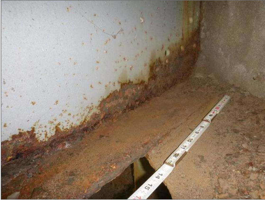
Span 3 Beam 3: [MUNICIPAL PROMPT ACTION REQUEST] AT END BENT 2, CORROSION WITH SECTION LOSS: BOTTOM FLANGE (0.38" AVERAGE REMAINING X 4.5'); LOWER WEB (1/4" AVERAGE REMAINING X 5' X UP TO 3")
