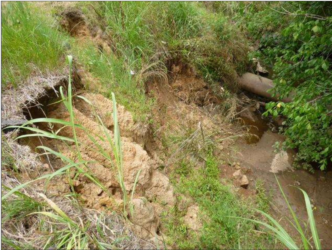
[MUNICIPAL PROMPT ACTION REQUEST] NORTHEAST CORNER IN THE FILL SLOPE, EROSION IS PRESENT, REACHING AS CLOSE AS 4' FROM THE EDGE OF PAVEMENT [APPROXIMATELY 40' LONG X UP TO 10' WIDE X UP TO 10' HIGH]
