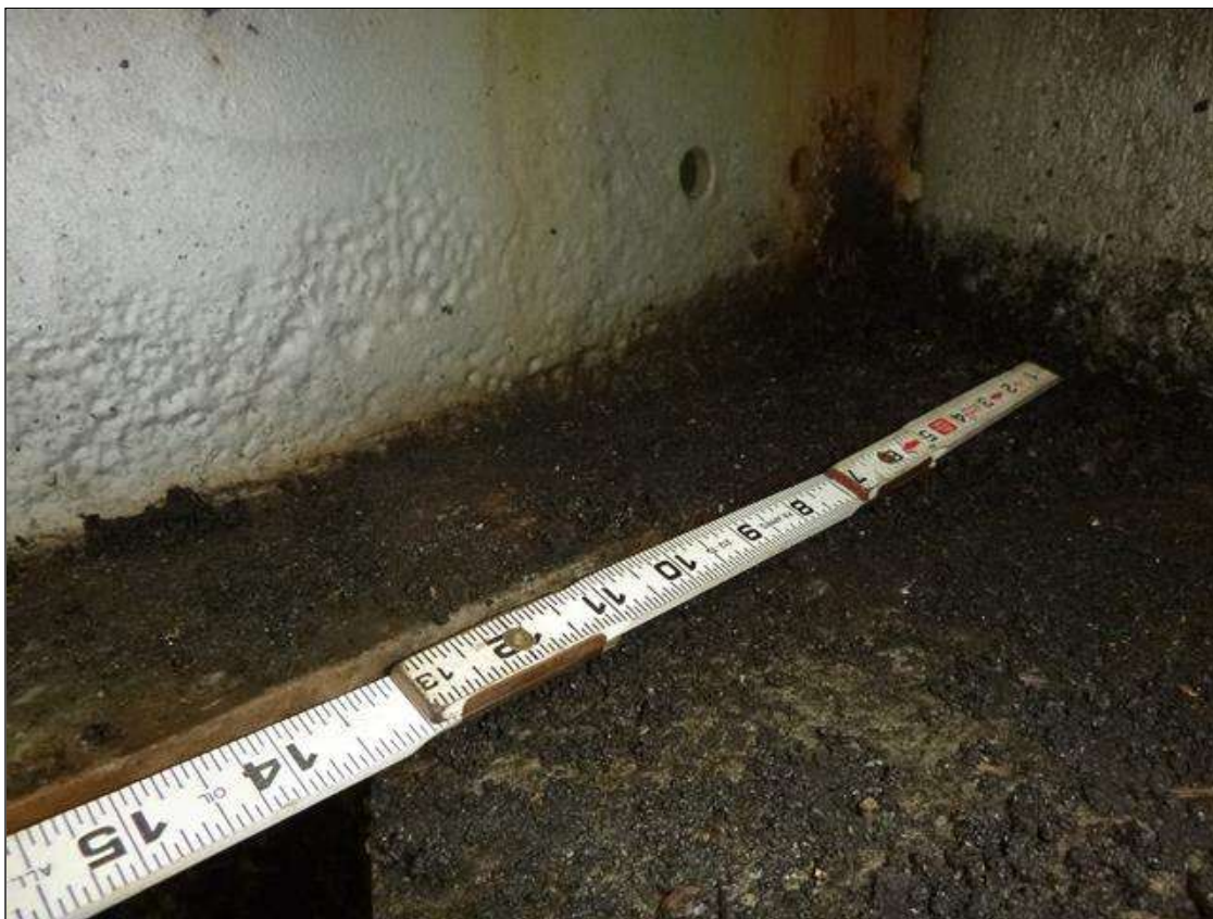
Span 1 Beam 1: [MUNICIPAL PROMPT ACTION REQUEST] at end bent 1, east face, corrosion with section loss: bottom flange (0.47" average remaining x 15"); lower web (1/4" average remaining x 27" x 2")
