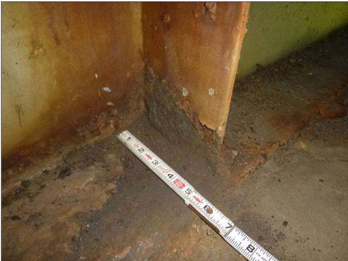
End Bent 1 Steel Cap 1: [MUNICIPAL PROMPT ACTION REQUEST] NORTH FACE IN THE THIRD WEB STIFFENER, LOWER 3", CORROSION WITH SECTION LOSS [AVERAGE 1/8" REMAINING].
