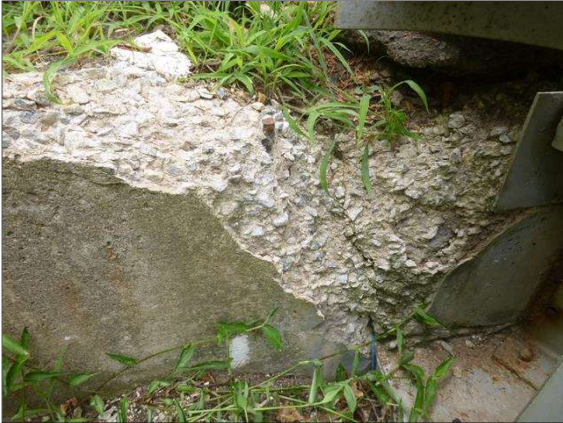
End Bent 1 Abutment: [MUNICIPAL PROMPT ACTION REQUEST] SOUTHEAST WINGWALL ADJACENT TO CURB, SPALL (2.5' X 1.5' X 3" DEEP) WITH EXPOSED RUSTED REBAR. THE CONCRETE SHOWS SIGNS OF ALKALAI SILICA REACTION.
