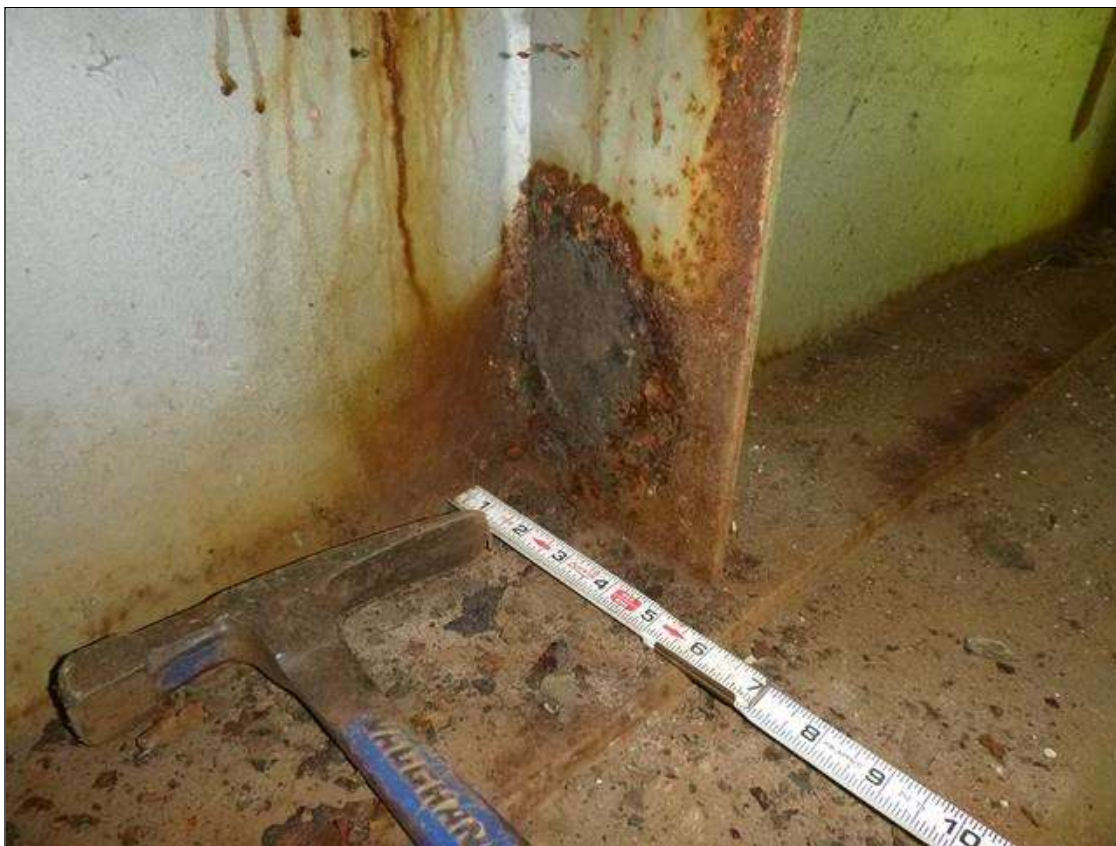
End Bent 2 Steel Cap 1: [MUNICIPAL PROMPT ACTION REQUEST] south face, web stiffener below beam 9, corrosion with section loss (0.20" average remaining x 4" x 5")
