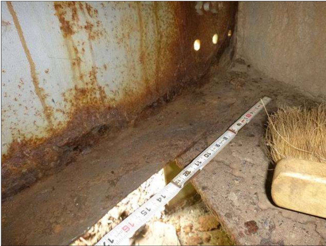
Span 1 Beam 10: [MUNICIPAL PROMPT ACTION REQUEST] AT END BENT 1, WEST FACE, CORROSION WITH SECTION LOSS: BOTTOM FLANGE (0.37" AVERAGE REMAINING X 2.5'); LOWER WEB (5/16" AVERAGE REMAINING X 3' X UP TO 4"); TOP FLANGE (0.38" AVERAGE REMAINING X 5')
