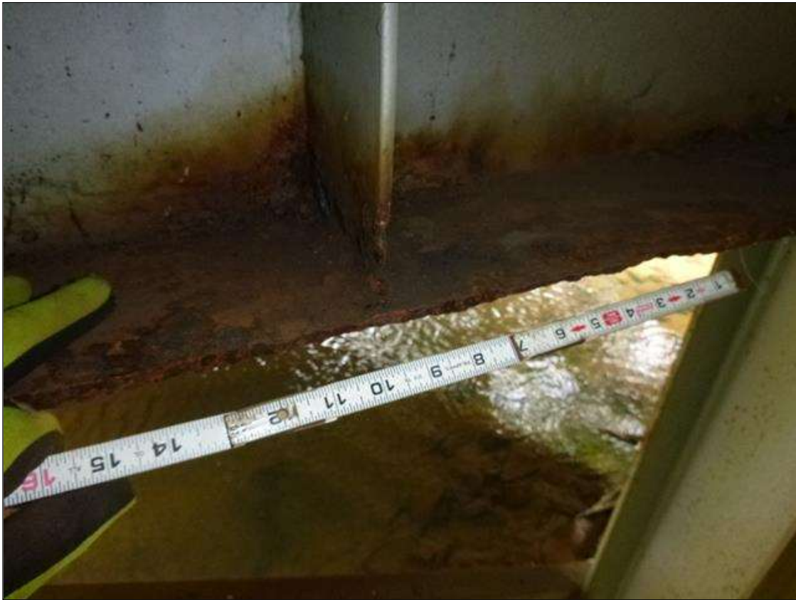
Bent 1 Cap 1: [MUNICIPAL PROMPT ACTION REQUEST] south face below beam 2, corrosion with section loss: bottom flange (0.35" average remaining x 2') top flange (0.42" average remaining x 1'); lower web (7/16" average remaining 2.5' x 2"); web stiffener (3/16" average remaining 5" x 2")
