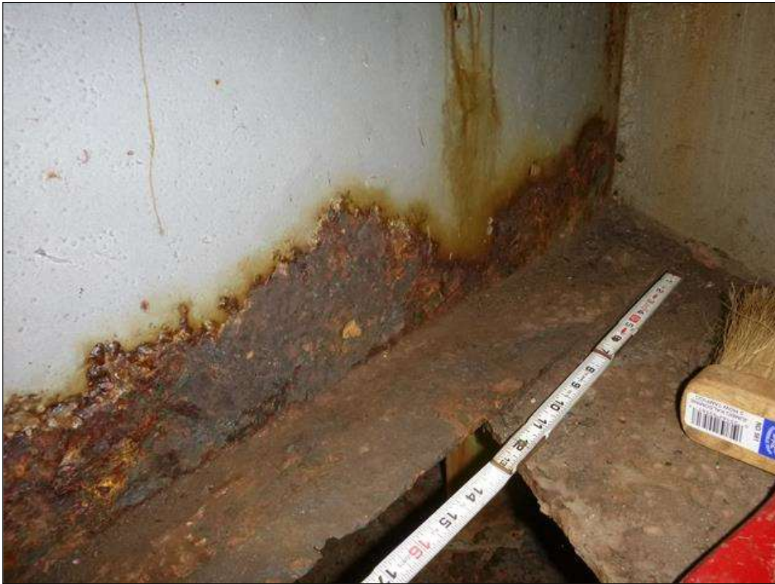
Span 1 Beam 2: [MUNICIPAL PROMPT ACTION REQUEST] AT END BENT 1, CORROSION WITH SECTION LOSS: BRT OTTOM FLANGE (0.40" AVERAGE REMAINING X 4'); LOWER WEB (1/4" AVERAGE REMAINING X 4' X UP TO 4") ; LEFT BOTTOM FLANGE CORROSION [AVERAGE 1/4" REMAINING] WITH KNIFE EDGING FOR 3' LONG.
