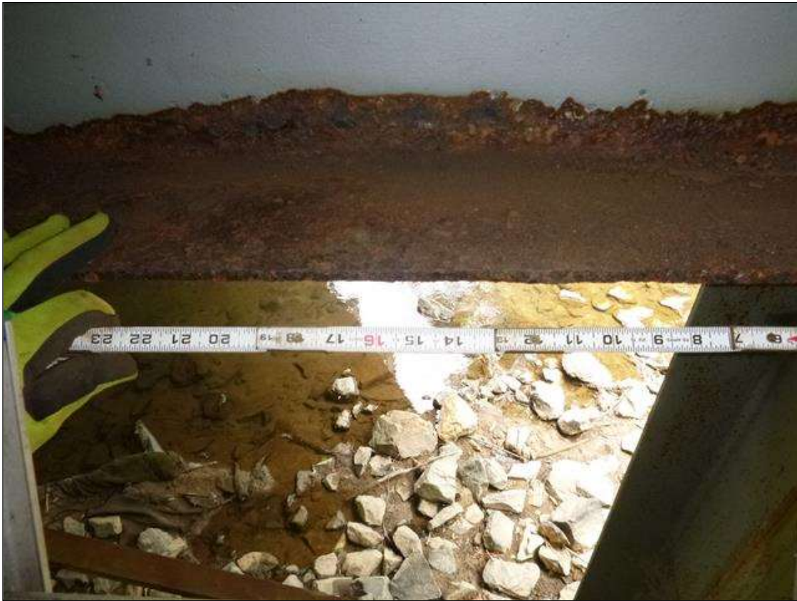
Bent 1 Cap 1: [MUNICIPAL PROMPT ACTION REQUEST] south and north faces below bays 7 through 9, corrosion with section loss: bottom flange (5/16" average remaining x 8.5'); lower web (7/16" average remaining x 8' x 2"); web stiffeners (as little as 0.15" average remaining x 5" x up to 5")
