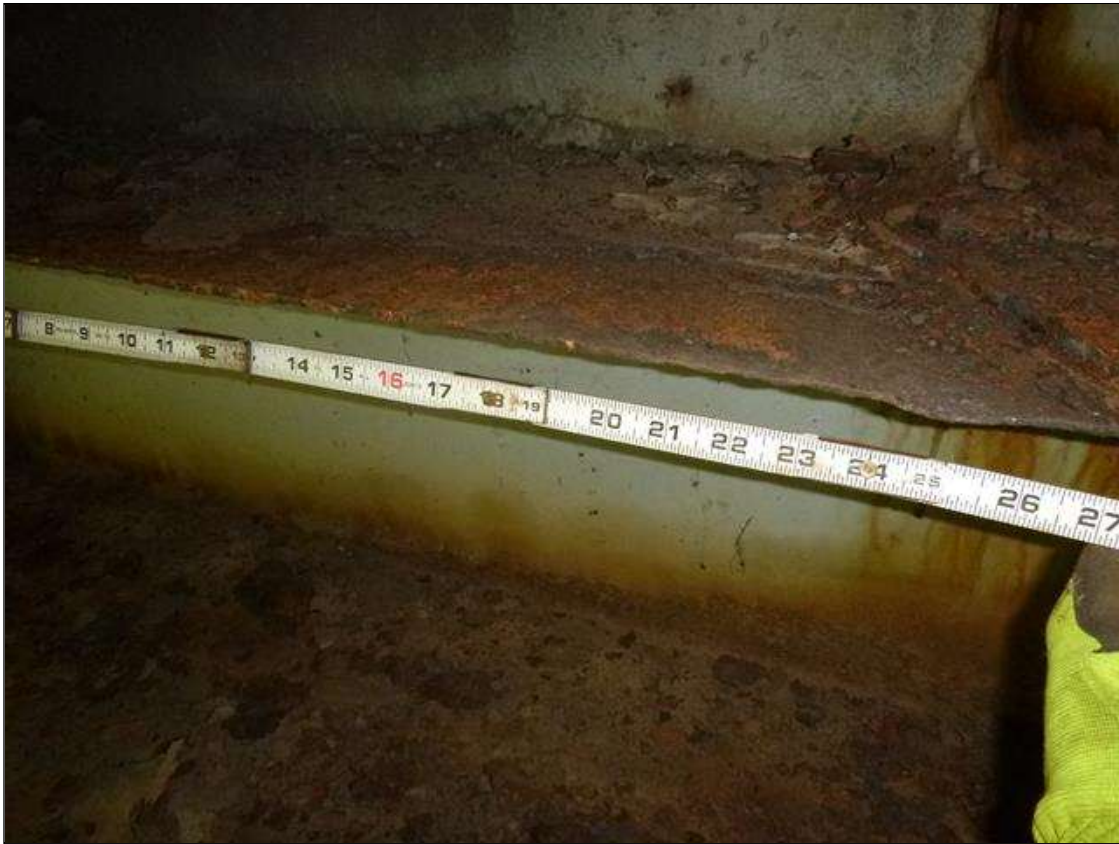
End Bent 2 Steel Cap 1: [MUNICIPAL PROMPT ACTION REQUEST] south face of cap in bays 3 and 4, corrosion with section loss: top flange (3/16" average remaining x 5.5' x 5"); lower web (7/16" average remaining x 4' x up to 2.5"); bottom flange (7/16" average remaining x 4.5'); web stiffeners (as little as 0.22" average remaining x 5" x up to full height)
