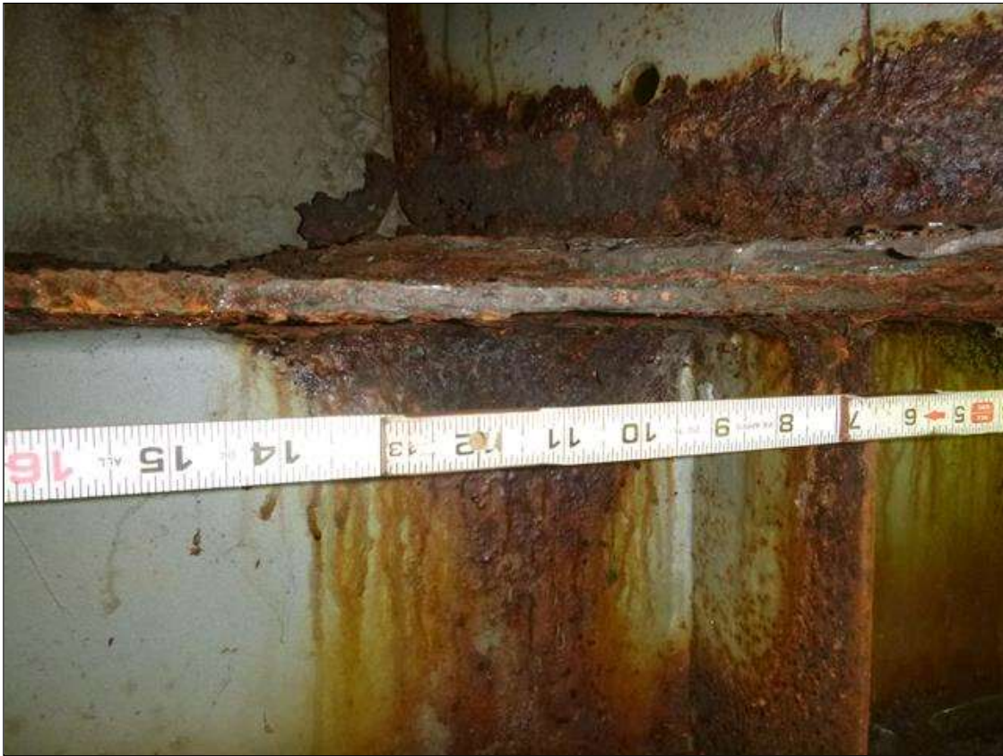
End Bent 2 Steel Cap 1: [MUNICIPAL PROMPT ACTION REQUEST] south face of cap below beam 8, corrosion with section loss: top flange (0.29" average remaining x 18" x 5"); upper web (7/16" average remaining x 6" x 2.5"); web stiffener (0.25" average remaining x 5" x 1")
