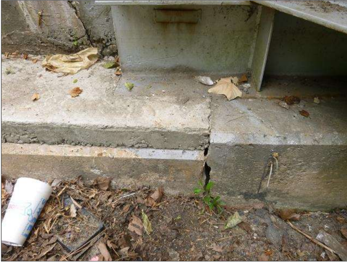
End Bent 2 Concrete Cap 1: [MUNICIPAL PROMPT ACTION REQUEST] west end of concrete cap, fracture (1' long x full width) undermining steel cap (1' long x 2" high x 1' deep)
