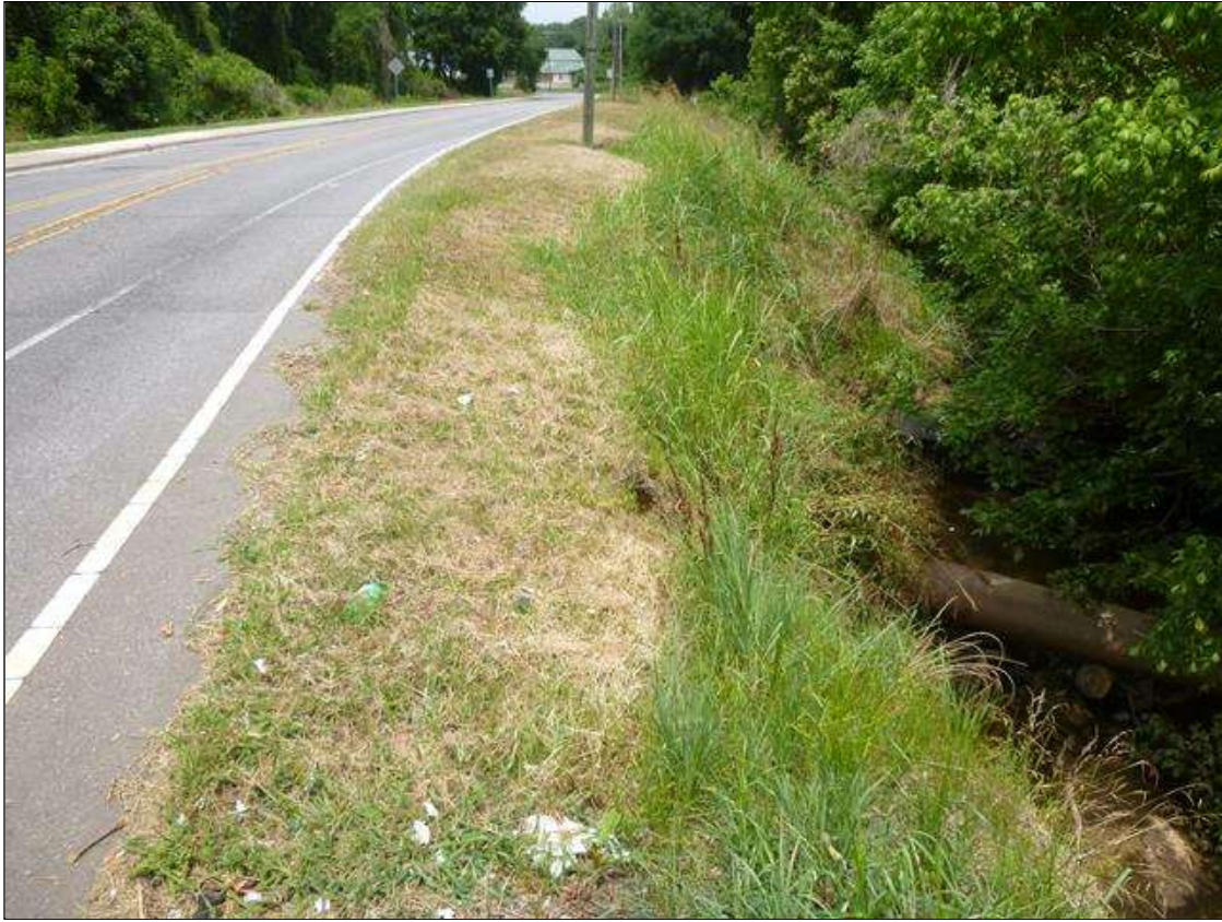
[MUNICIPAL PROMPT ACTION REQUEST] NORTHEAST CORNER IN THE FILL SLOPE, EROSION IS PRESENT, REACHING AS CLOSE AS 4' FROM THE EDGE OF PAVEMENT [APPROXIMATELY 40' LONG X UP TO 10' WIDE X UP TO 10' HIGH]
