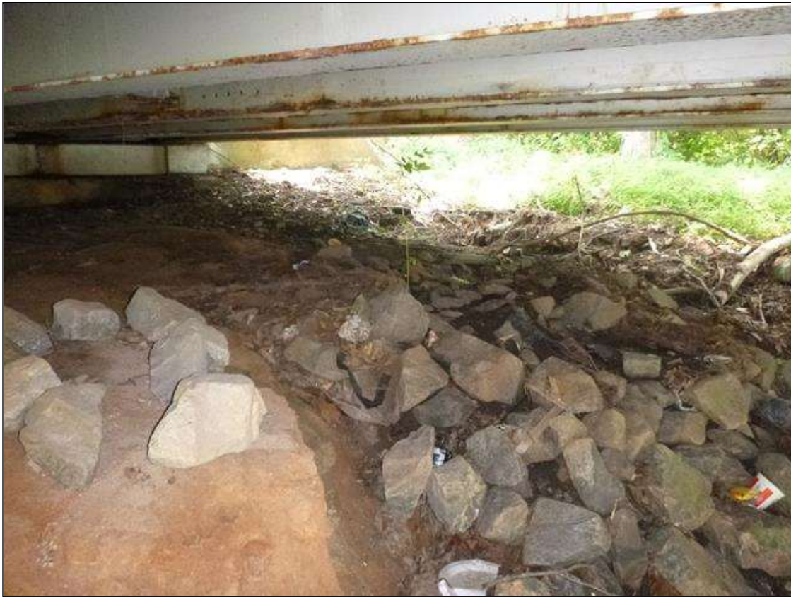
[MUNICIPAL PROMPT ACTION REQUEST] AT ABUTMENT 1 IN THE TOP OF THE SLOPE, RIGHT & LEFT SIDES, SCATTERED EROSION [APPROXIMATELY 160 SQUARE FEET TOTAL X UP TO 1.25' DEEP]
