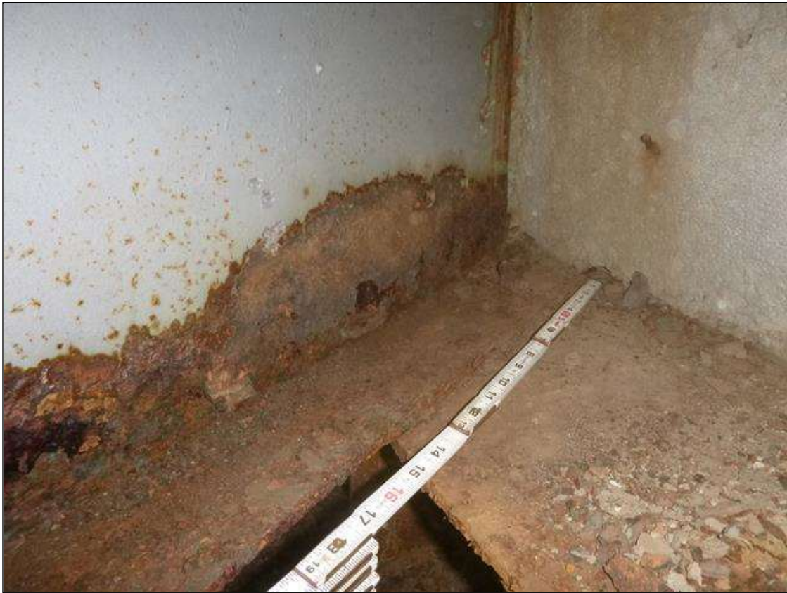
Span 3 Beam 7: [MUNICIPAL PROMPT ACTION REQUEST] AT END BENT 2, CORROSION WITH SECTION LOSS: BOTTOM FLANGE (0.42" AVERAGE REMAINING X UP TO 5.5'); LOWER WEB (3/16" AVERAGE REMAINING X 5.5' X UP TO 4")
