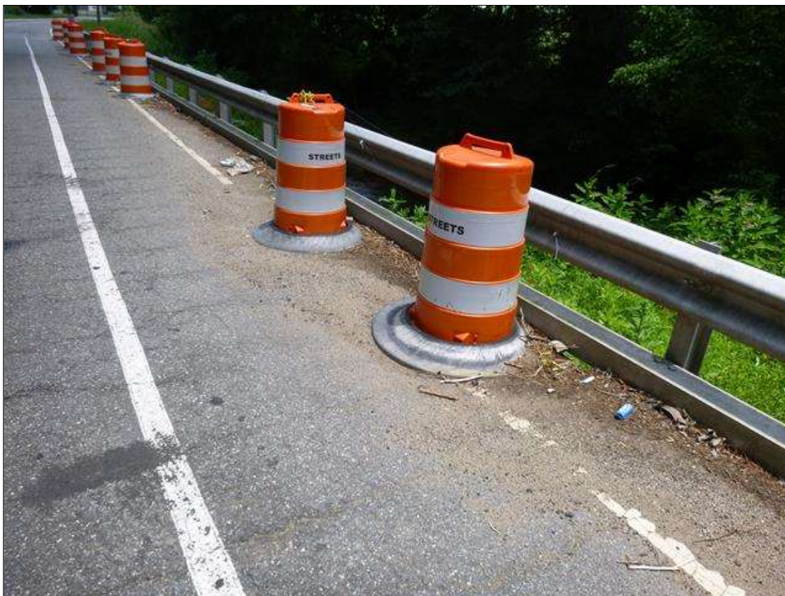
RIGHT AND LEFT GUTTERLINES, DEBRIS ACCUMULATION ALONG THE LENGTHS
