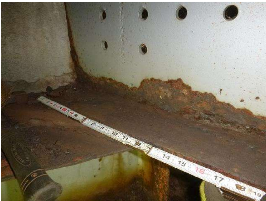
Span 3 Beam 5: [MUNICIPAL PROMPT ACTION REQUEST] AT END BENT 2, CORROSION WITH SECTION LOSS: BOTTOM FLANGE (3/8" AVERAGE REMAINING X 3'); LOWER WEB (3/16" AVERAGE REMAINING X 3.5' X UP TO 3')
