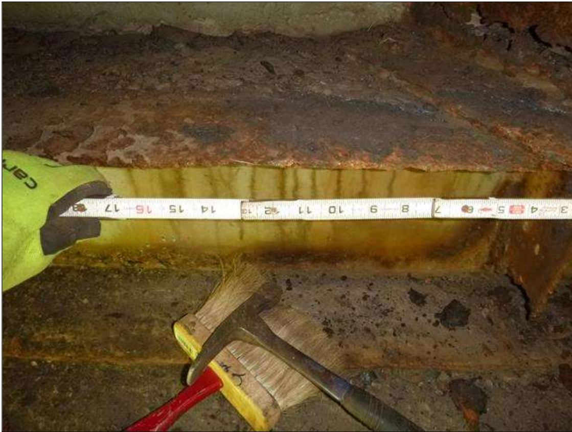
End Bent 1 Steel Cap 1: [MUNICIPAL PROMPT ACTION REQUEST] NORTH TOP FLANGE EAST OF BEAM 8, CORROSION WITH SECTION LOSS (0.28" AVERAGE REMAINING X 1.5' X 4")
