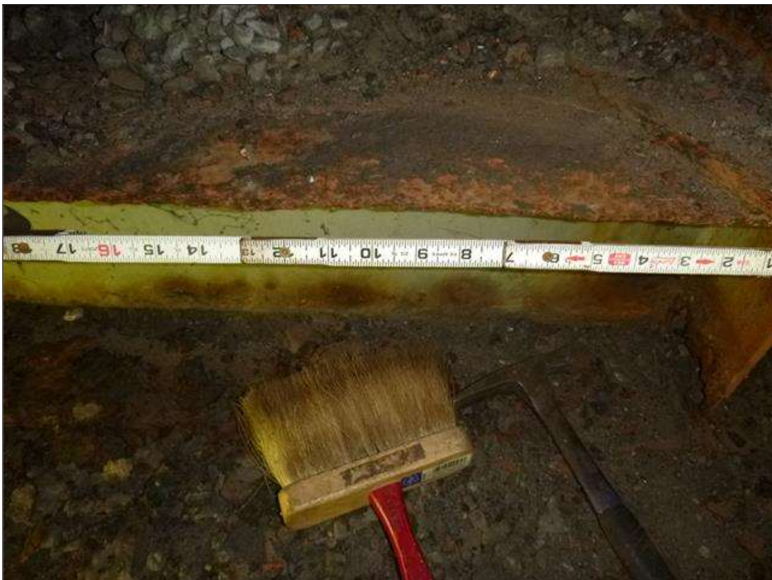
End Bent 1 Steel Cap 1: [MUNICIPAL PROMPT ACTION REQUEST] NORTH TOP FLANGE EAST OF BEAM 7, CORROSION WITH SECTION LOSS (0.28" AVERAGE REMAINING X 18" X 5")
