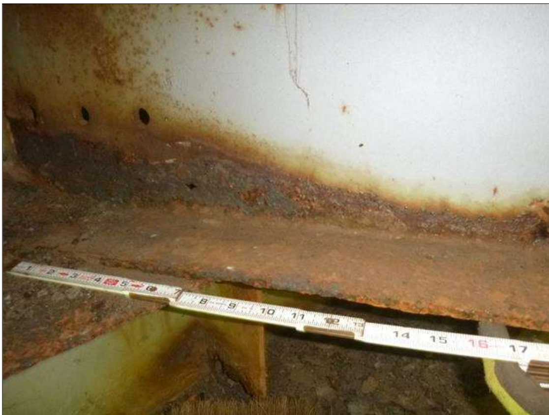
Span 1 Beam 7: [MUNICIPAL PROMPT ACTION REQUEST] AT END BENT 1, CORROSION WITH SECTION LOSS: BOTTOM FLANGE (0.45" AVERAGE REMAINING X 4.5'); LOWER WEB (1/4" AVERAGE REMAINING X 4.5' X UP TO 4" WITH 1" DIAMETER CORROSION HOLE AT 1' OUT).
