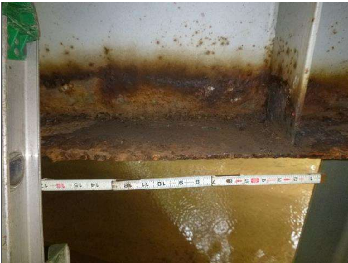
Bent 2 Cap 1: [MUNICIPAL PROMPT ACTION REQUEST] north face below bays 4 through 6, corrosion with section loss: bottom flange (0.33" average remaining x 5.5" x 9"); lower web (less than 1/16" loss x 9' x 2"); web stiffeners in the lower 2", average 3/16" remains.
