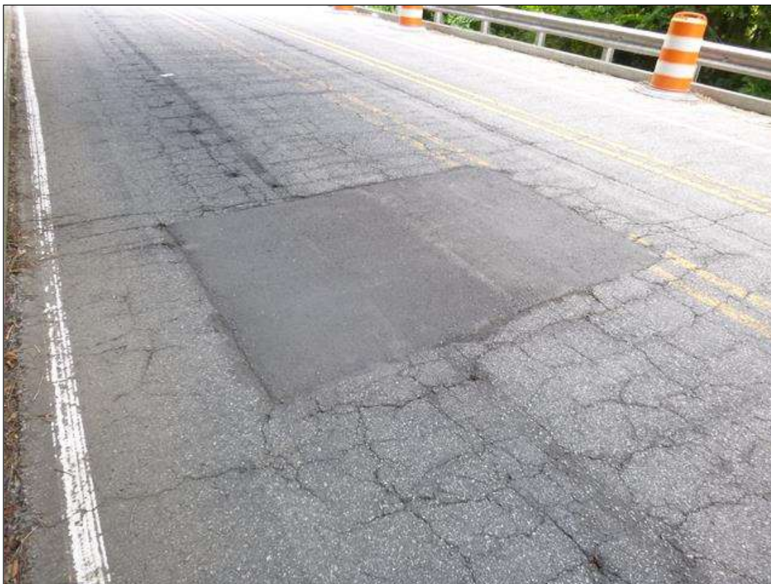
Span 1 Wearing Surface: [NEW REPAIR - ASPHALT PATCHING] FORMERLY --> at southbound lane adjacent to bent 1, patched area (4.5' x 4') with cracks (up to 1/8") and potholes (up to 2" x 3" x 1" deep)
