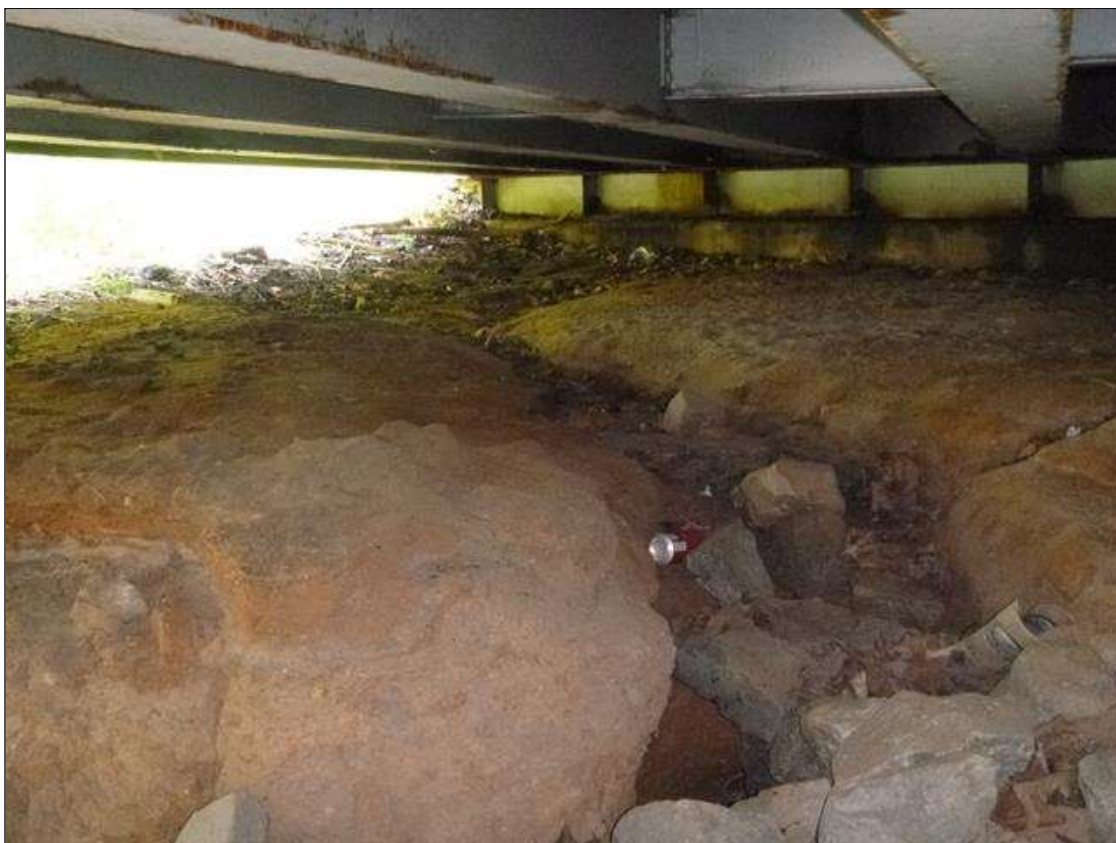
[MUNICIPAL PROMPT ACTION REQUEST] AT ABUTMENT 1 IN THE TOP OF THE SLOPE, RIGHT & LEFT SIDES, SCATTERED EROSION [APPROXIMATELY 160 SQUARE FEET TOTAL X UP TO 1.25' DEEP]
