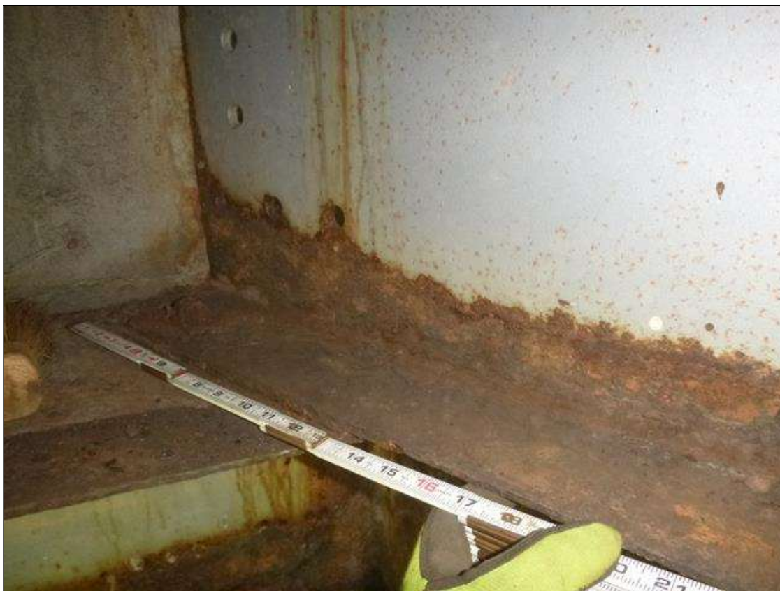
Span 3 Beam 6: [MUNICIPAL PROMPT ACTION REQUEST] AT END BENT 2, CORROSION WITH SECTION LOSS: BOTTOM FLANGE (0.35" AVERAGE REMAINING X 6'); LOWER WEB (3/16" AVERAGE REMAINING X 6' X UP TO 4")
