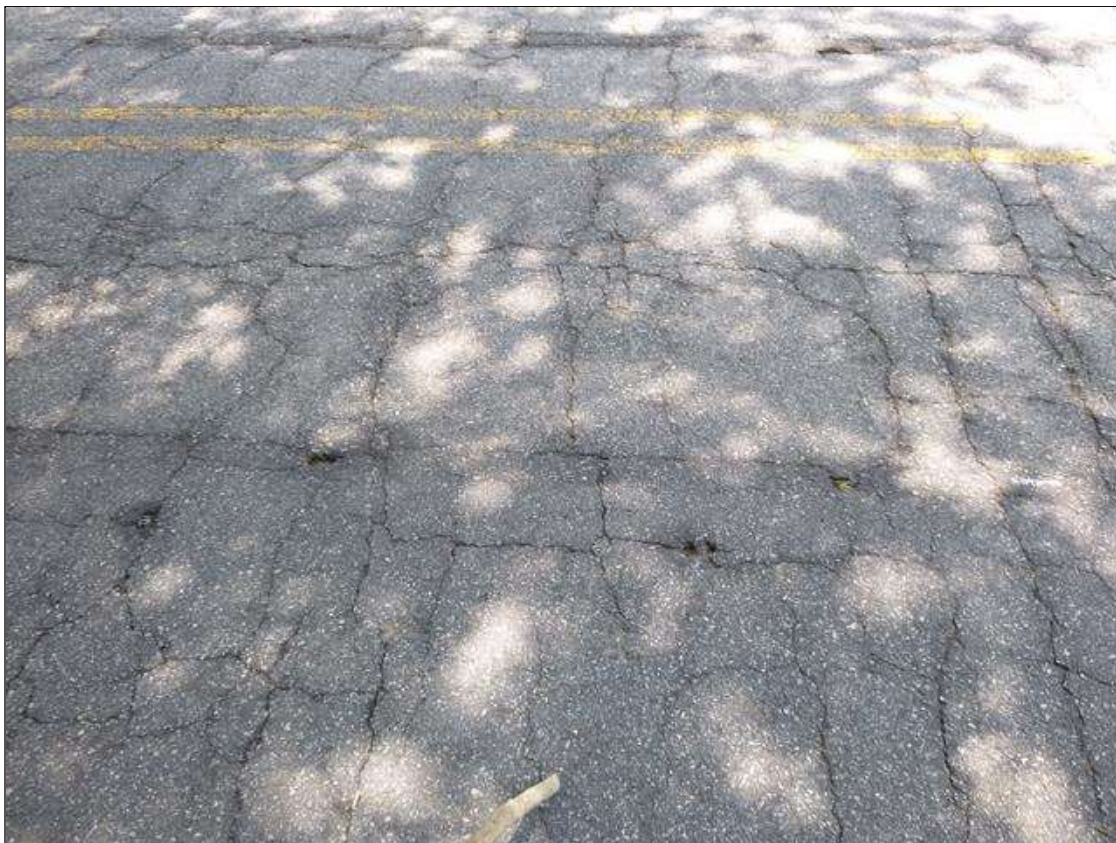
Span 1 Wearing Surface: throughout wearing surface, map cracks (up to 1/2" x full width of roadway x full length)
