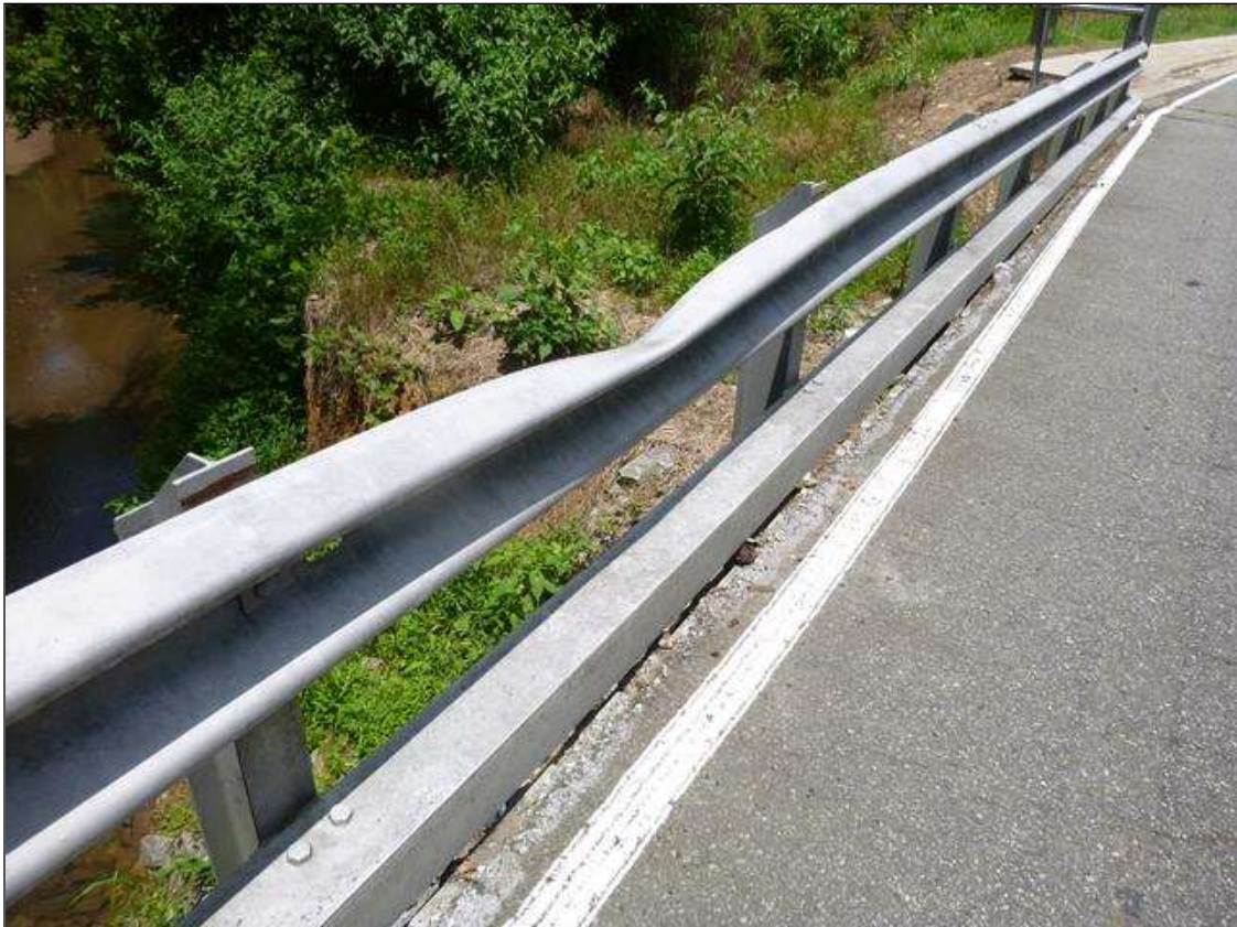
Span 3 Left Bridge Rail: left bridge rail at 18' from end bent 2, impact damage (2')
