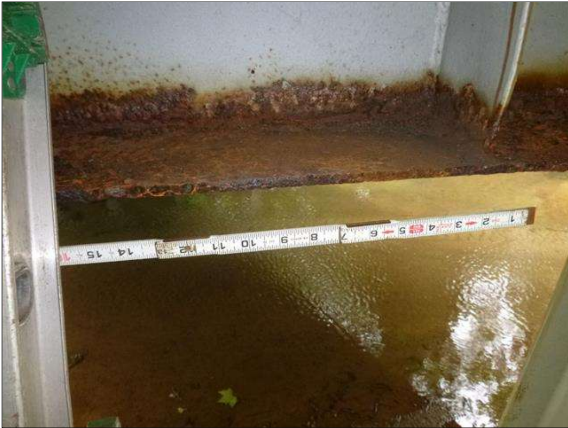
Bent 2 Cap 1: [MUNICIPAL PROMPT ACTION REQUEST] north face below bay 7, corrosion with section loss: bottom flange (0.35" average remaining x 5.5" x 3.5'); top flange (0.35" average remaining x 5.5" x 3.5'); lower web (less than 1/16" loss x 3.5' x 2"); web stiffeners (less than 1/16" loss x 5" x 2")
