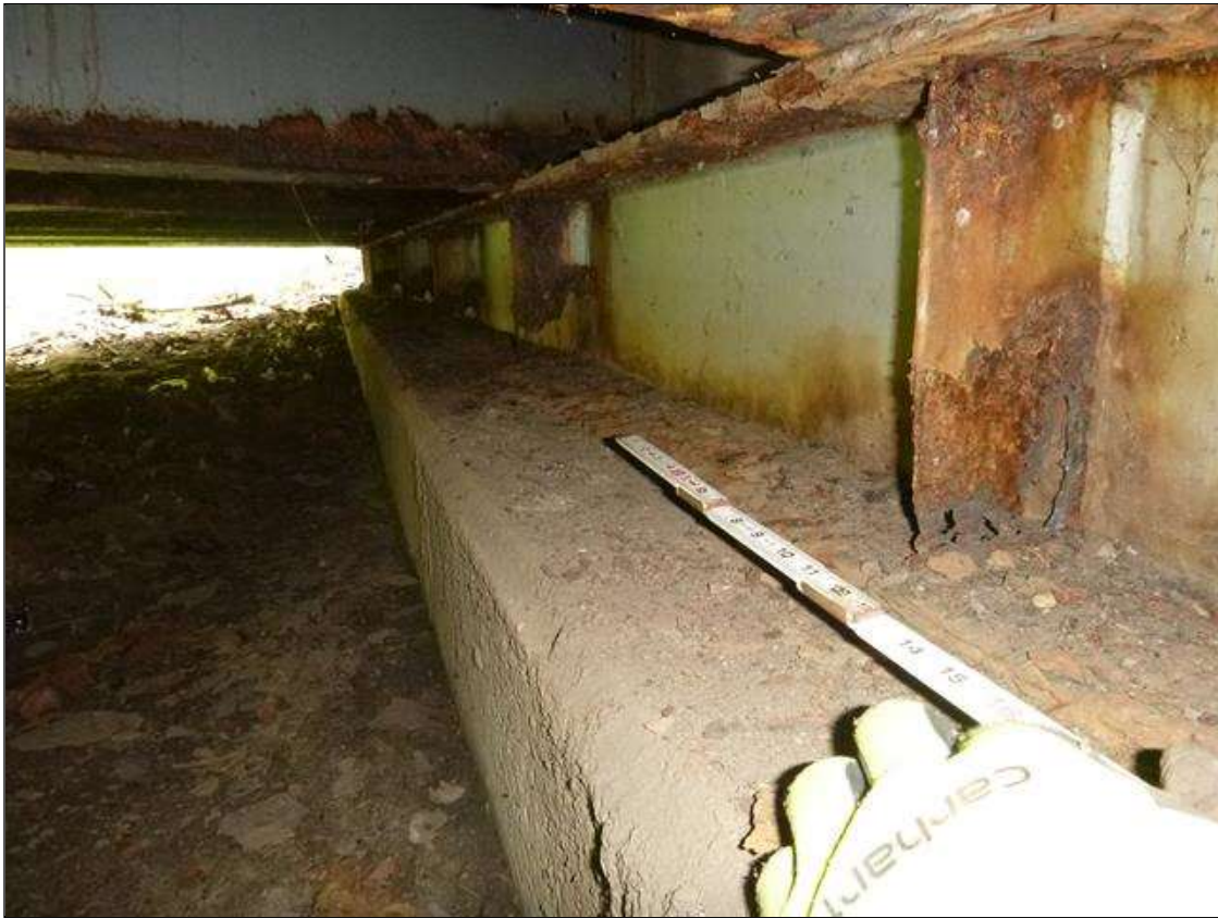
End Bent 1 Steel Cap 1: [MUNICIPAL PROMPT ACTION REQUEST] NORTH FACE IN THE LOWER 3" OF WEB STIFFENERS 4-9, CORROSION WITH 100% SECTION LOSS.
