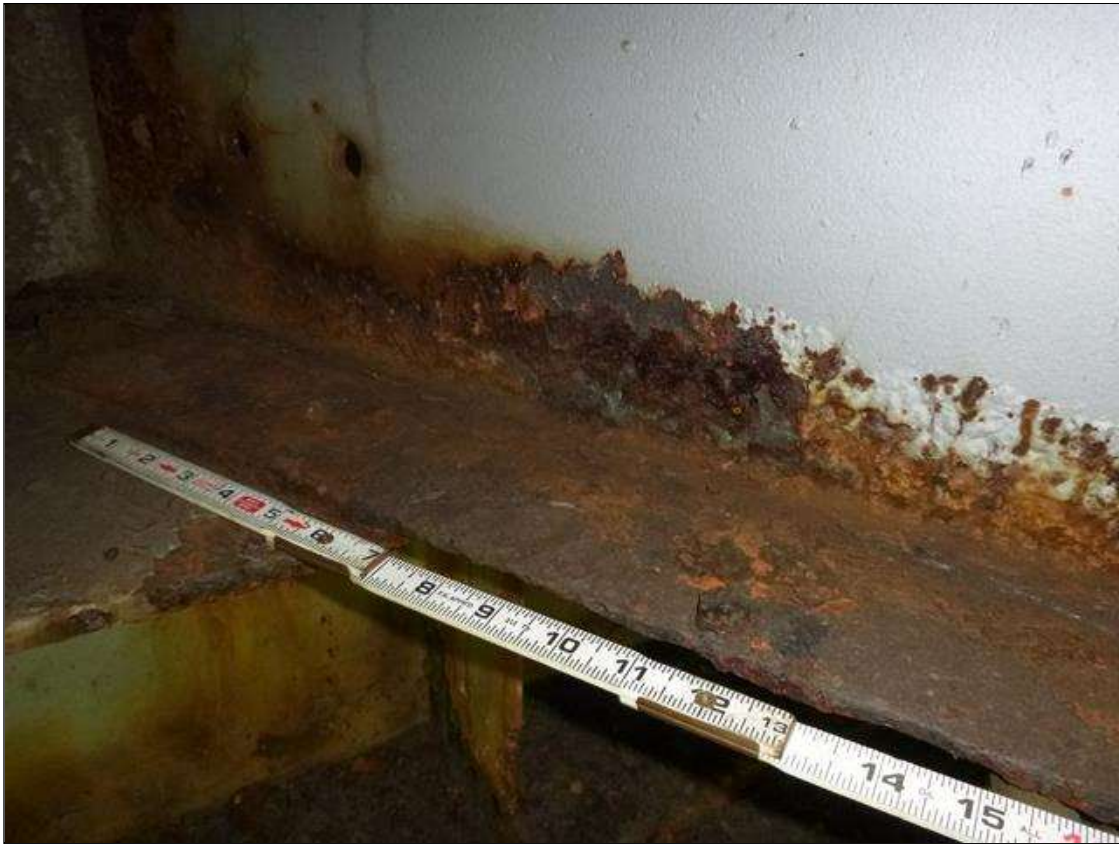
Span 1 Beam 4: [MUNICIPAL PROMPT ACTION REQUEST] AT END BENT 1, CORROSION WITH SECTION LOSS: LEFT BOTTOM FLANGE (0.47" AVERAGE REMAINING X 50"), RIGHT BOTTOM FLANGE (1/4" AVERAGE REMAINING FOR 1.5' LONG, THEN 0.47" AVERAGE REMAINING FOR NEXT 2.5' LONG); LOWER WEB (1/4" AVERAGE REMAINING X 4' X UP TO 4")
