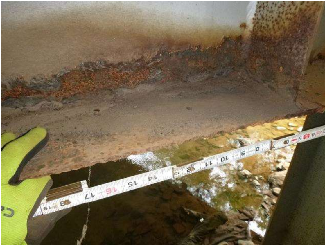
Bent 1 Cap 1: [MUNICIPAL PROMPT ACTION REQUEST] south face below bay 3, corrosion with section loss: bottom flange (1/4" average remaining x 39"); lower web (7/16" average remaining x 39" x 2"); web stiffeners (as little as 3/16" average remaining x 5" x 2.5")
